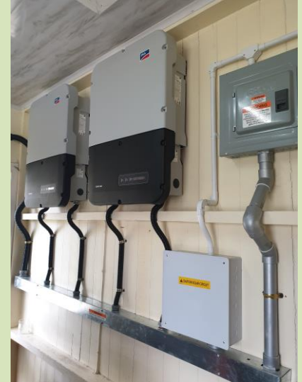
Grid Connected Inverter System @ Public Building
