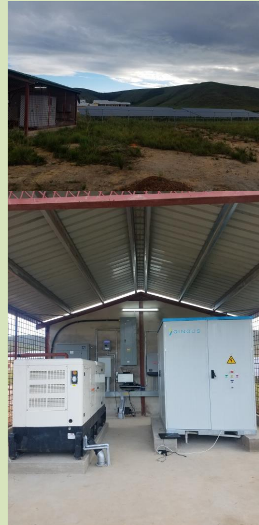
Complete Micro Grid Solar PV System w/ BESS Installed @ Kato
