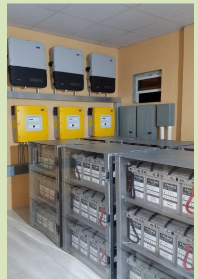
Large Battery Energy Storage System Installed @ MoPI
