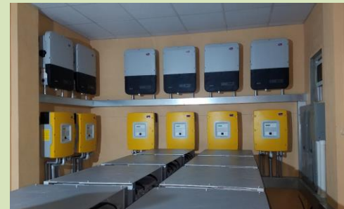
AC Coupled System with Frequency Shifting Capability Installed @ MoPI
