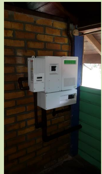
Typical Medium Size Inverter System Installation with BoS Components
