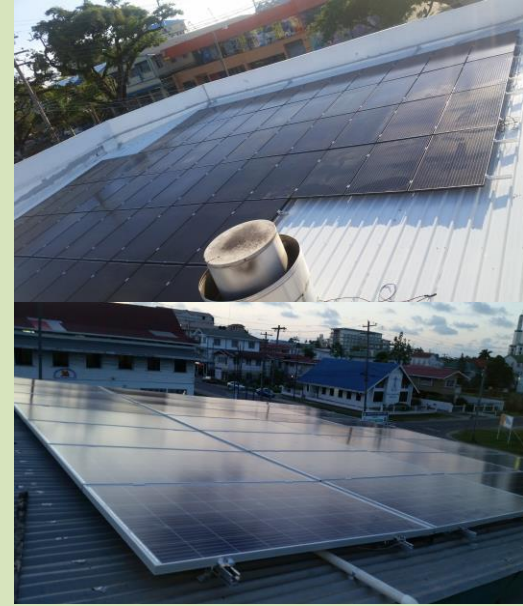
PV Array @ Banks DIH. On Grid System with Load Management Capability. PV System powers load during a grid failure.
