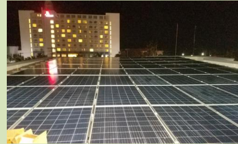
34 kW Solar Array Installed on Flat Concrete Roof @ MoPI
