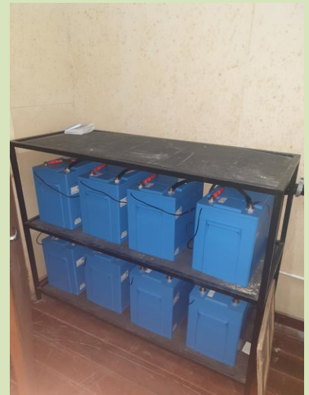
Lithium Iron Phosphate Battery Bank
