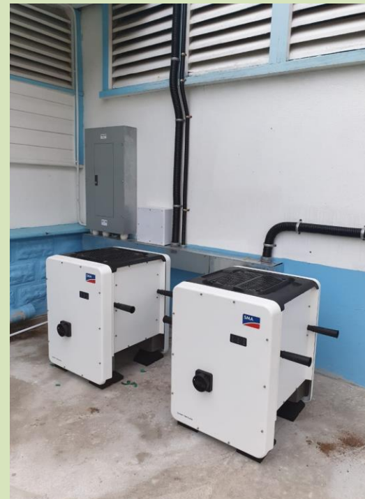
On Grid Inverters for 100 kW System @ University of Guyana
