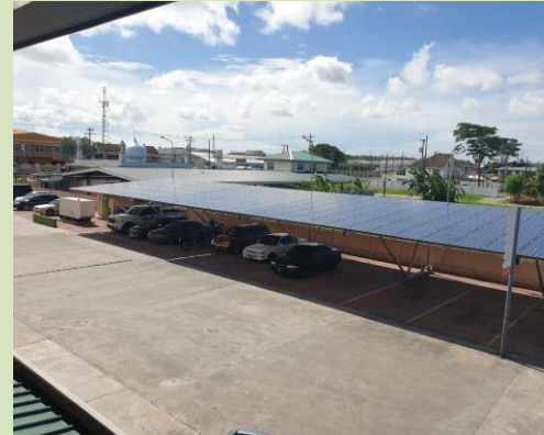
Solar PV Carport Installed at our Head Office
