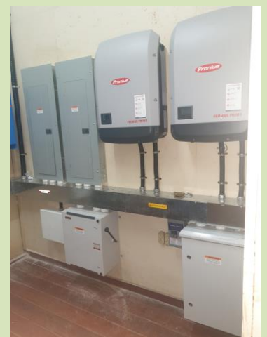
Typical PV Inverter Installation
