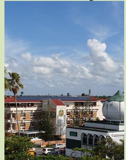
PV Array Installed @ NIS
