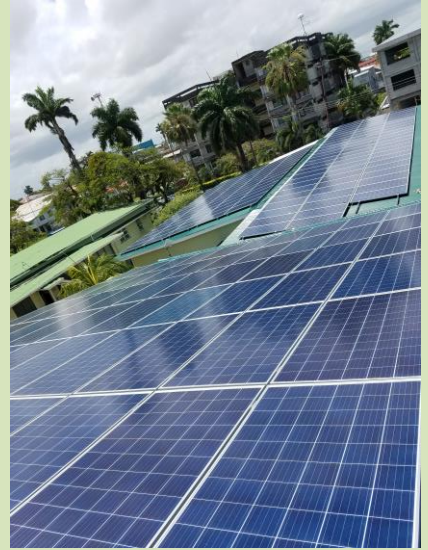
130kW PV Array Installed @ Ministry of the Presidency
