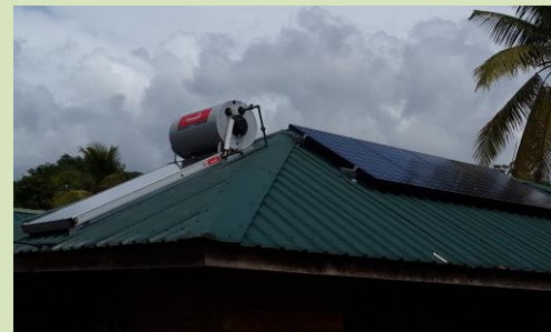
Small Solar PV Array and Solar Water Heater Installed @ Iwokrama
